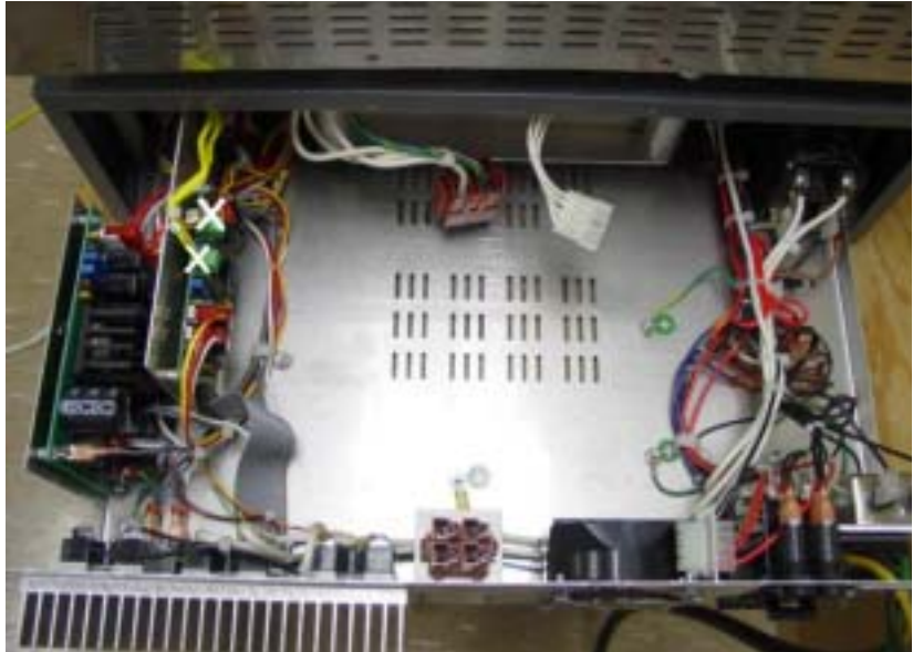
Control panel slid out 1/2 way
