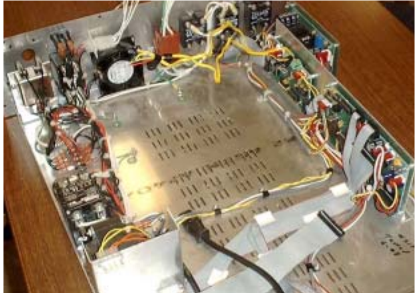
Control section pulled from unit
